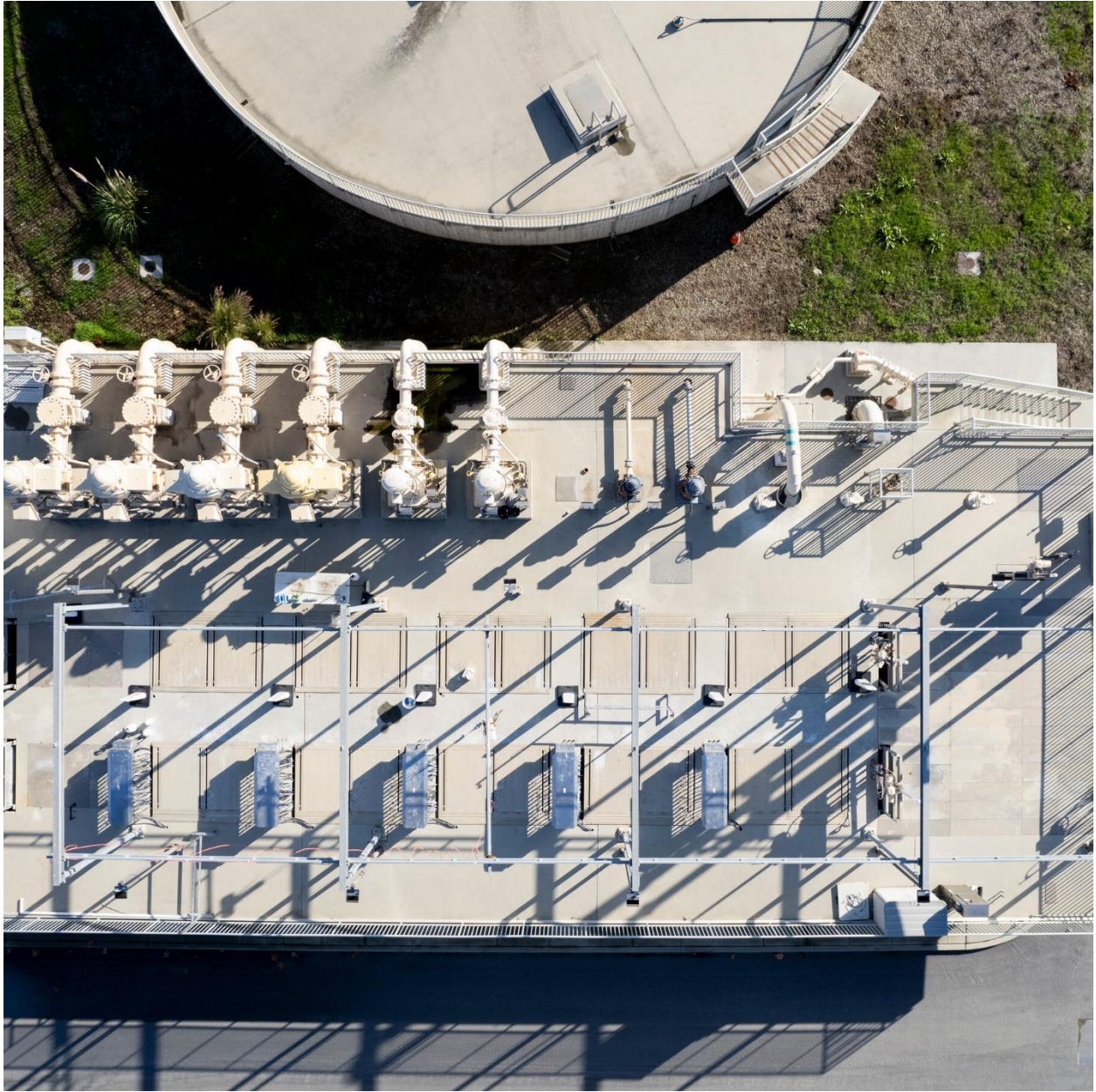
The Pajaro Valley water treatment center.
