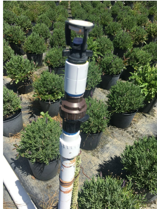
Sprinkler check valves
